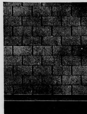
Reynolds Slate Shingles After Five Years Wear
