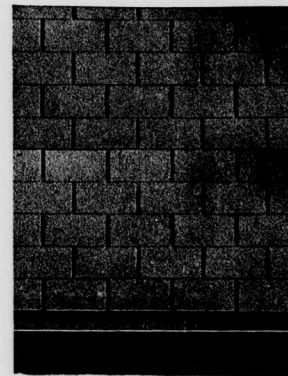
Reynolds Slate Shingles After Five Years Wear
