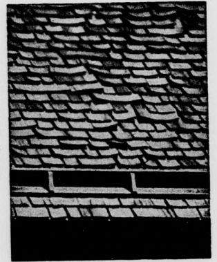
Wood Shingles After Five Years Wear
