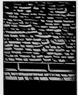
Wood Shingles After Five Years Wear
