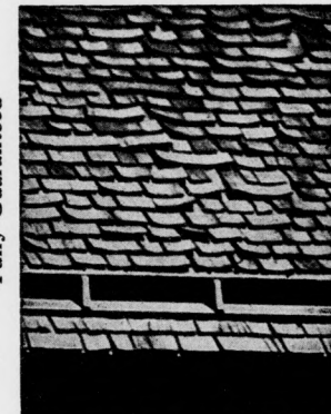
Wood Shingles After Five Years Wear
