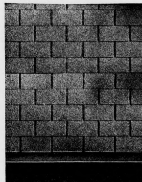
Reynolds Slate Shingles After Five Years Wear
