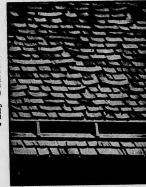
Wood Shingles After Five Years Wear
