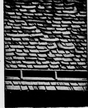
Wood Shingles After Five Years Wear
