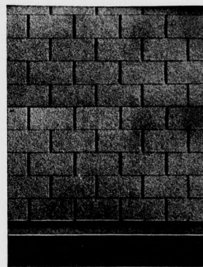
Reynolds Slate Shingles After Five Years Wear
