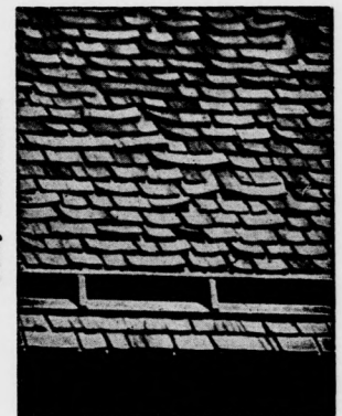
Wood Shingles After Five Years Wear
