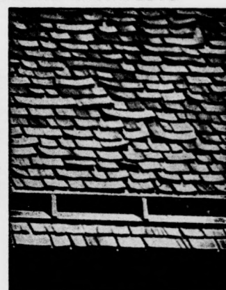
Wood Shingles After Five Years Wear
