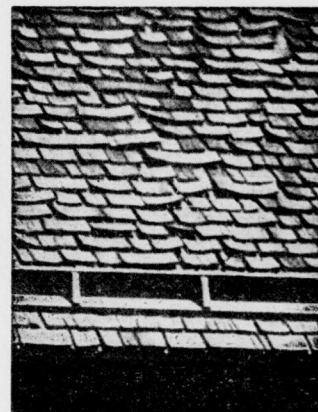
Wood Shingles After Five Years Wear
