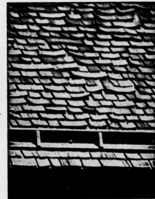
Wood Shingles After Five Years Wear
