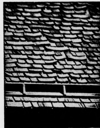
Wood Shingles After Five Years Wear
