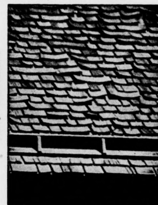
Wood Shingles After Five Years Wear
