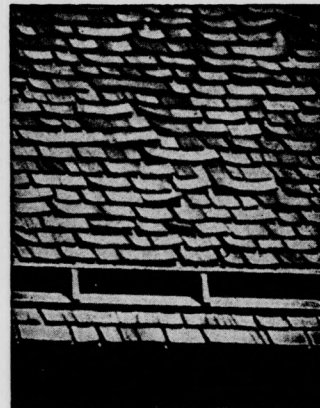
Wood Shingles After Five Years Wear
