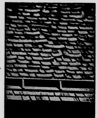
Wood Shingles After Five Years Wear
