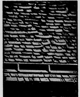
Wood Shingles After Five Years Wear
