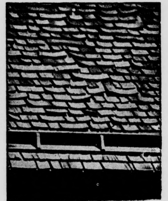
Wood Shingles After Five Years Wear
