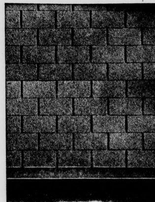
Reynolds Slate Shingles After Five Years Wear
