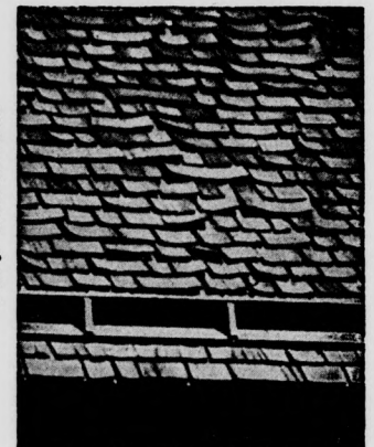
Wood Shingles After Five Years Wear
