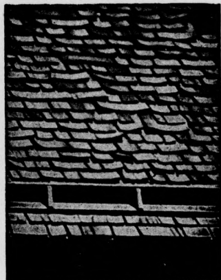
Wood Shingles After Five Years Wear
