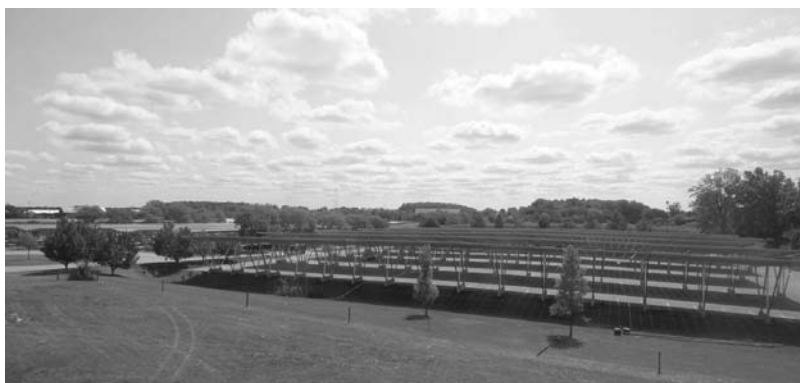
Construction progress as of August 25, 2017 on one of MSU's five commuter parking lots getting outfitted with a solar carport.
