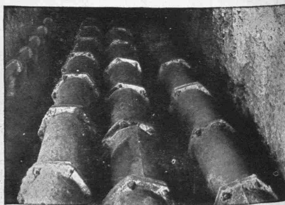
Section of 285-year-old cast iron water main still serving the town and fountains of Versailles, France.
