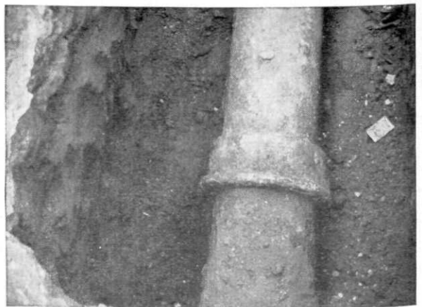
Cast iron water main still functioning in Philadelphia after 135 years of service.
