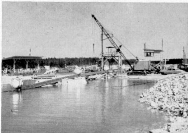
Here the pipe, with floats attached, is fed to the pulling cable, which attained a velocity of 20 feet per minute.
