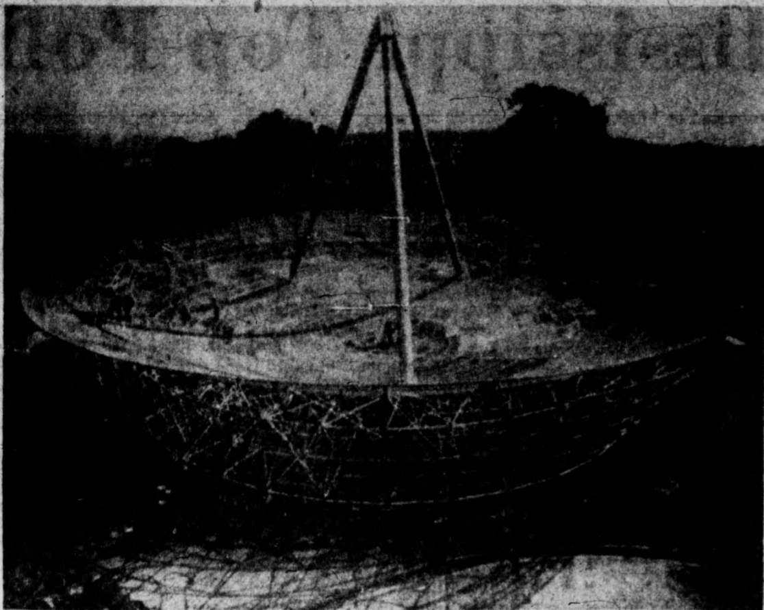
BIGGEST RADIO TELESCOPE DISH —Looking like ants in a saucer, workmen put the finishing touches on America's largest radio telescope "dish" on the Stanford University campus. Riggers are scheduled next week to lift the 70-ton, 150-foot steel aluminum antenna onto its mount. The antenna was designed and built by Stanford Research Institute scientists with support from the Air Force. MSU will clash with Stanford's football team this Saturday at the first home game. —AP Wirephoto.
