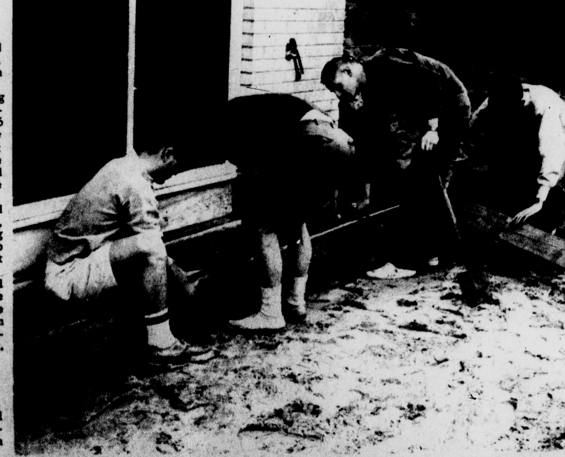
THE PATIO BUILDERS—Members of Delta Upsilon fraternity, 1504 E. Grand River, square-off cement forms prior to laying stone and concrete for a backyard patio. Warm weather, and a lack of relaxation area brought about the endeavor, according to fraternity members. —State News Photo by Mark Krastof.
