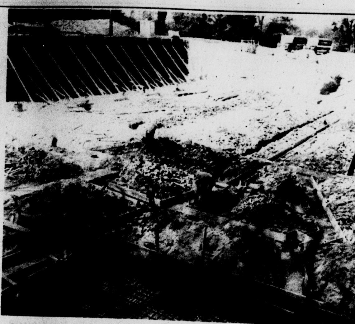
Construction is underway on the new $1.5 million University Methodist Church on Harrison Road. The structure is scheduled for completion early next year.
