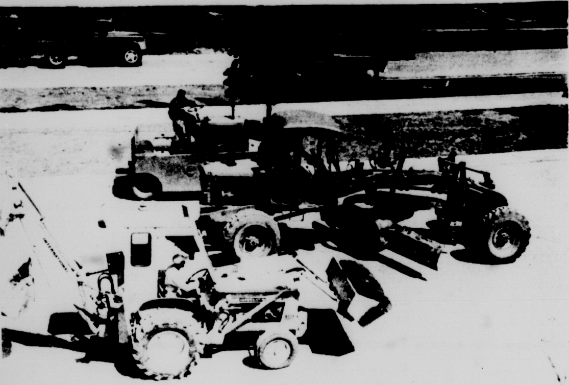
AND THEY'RE OFF--The green flag seems to have dropped on Bogue Street and the race to complete the construction project is on. Wait a minute. Is that Beetlebomb bringing up the rear? Photo by George Junne
