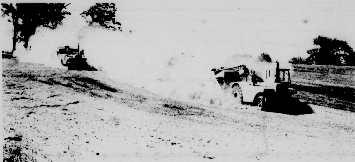
BITING THE DUST --That is what the driver of the second machine must be doing unless he is wearing a mask. However, it's just a part of the day's work in constructing parking lot Y at the corner of Farm Lane and Mt. Hope. Photo by Ken Roberts
