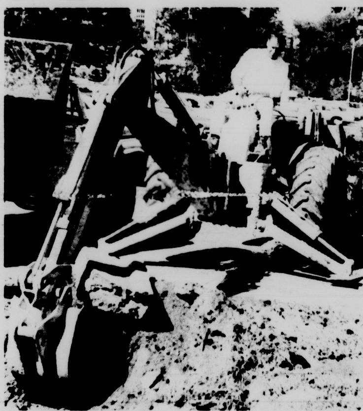
DIG THIS—Pictured is part of the work going on in front of the Home Management Building across from Student Services. So far there has been little word about the purpose of the work, but speculation is that it is concerned with the new bus system which will begin operation fall term.
