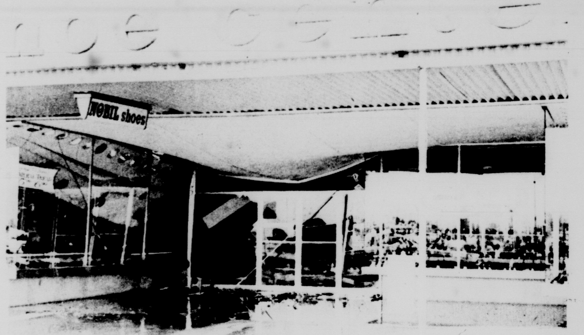
WEATHER AND LEATHER -- When these two meet, one is bound to win, and in this case the weather emerged the victor. This shoe store in the Logan Shopping Plaza was victimized when its roof, weighted down with water from Tuesday's downpour, could no longer support the load and collapsed. Photo by Larry Fritzman
