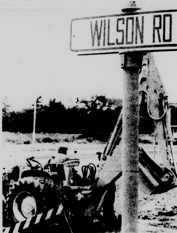
RIPPING AND TEARING -- It's all necessary, however, before traffic can travel on Wilson Road. But, until that time, construction crews continue to labor on the project. Photo by Ken Roberts
