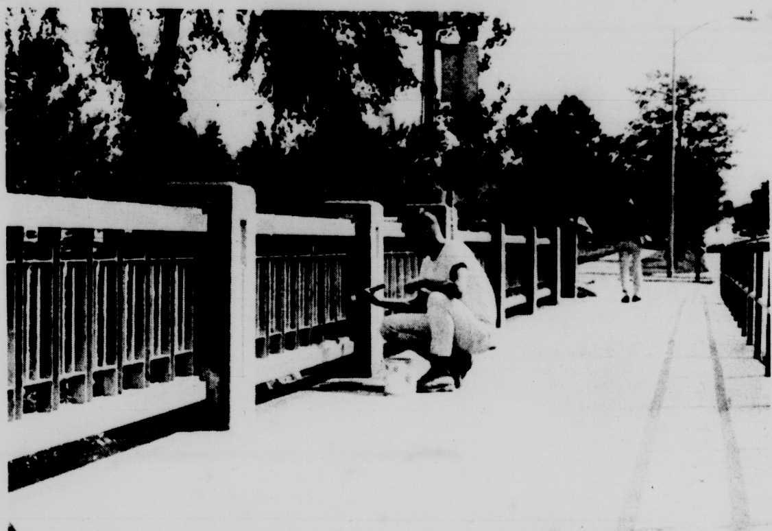
BRIDGE WORK -- Even the University's bridges get a summer fixing up. Here a workman paints the Farm Lane Bridge, heedless of the constant traffic which passes. Photo by Ken Roberts
