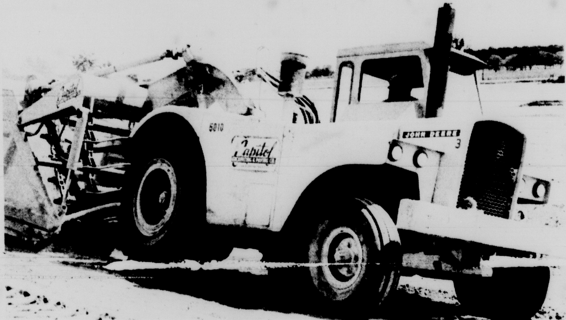
DEERE JOHN--With the opening of fall term only about a month away, work on Parking Lot Y, where commuters will park their vehicles, continues even on Saturdays. The driver, with his straw hat, looks like he's ready for a heavy date right after work. Photo by Larry Fritzlau
