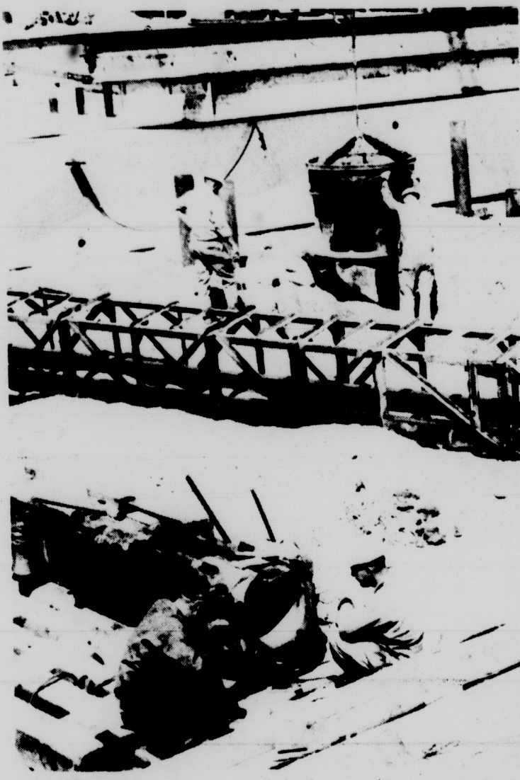
RELIEF CREW --This crew, which is working on construction of the new East Lansing Sewage Plant, will provide welcome relief for those who have suffered from the effects of "Brodyodor," so named because the odor is most noticeable near the Brody dormitories. The odor comes from the present sewage plant, located across the river from Bailey Hall.
