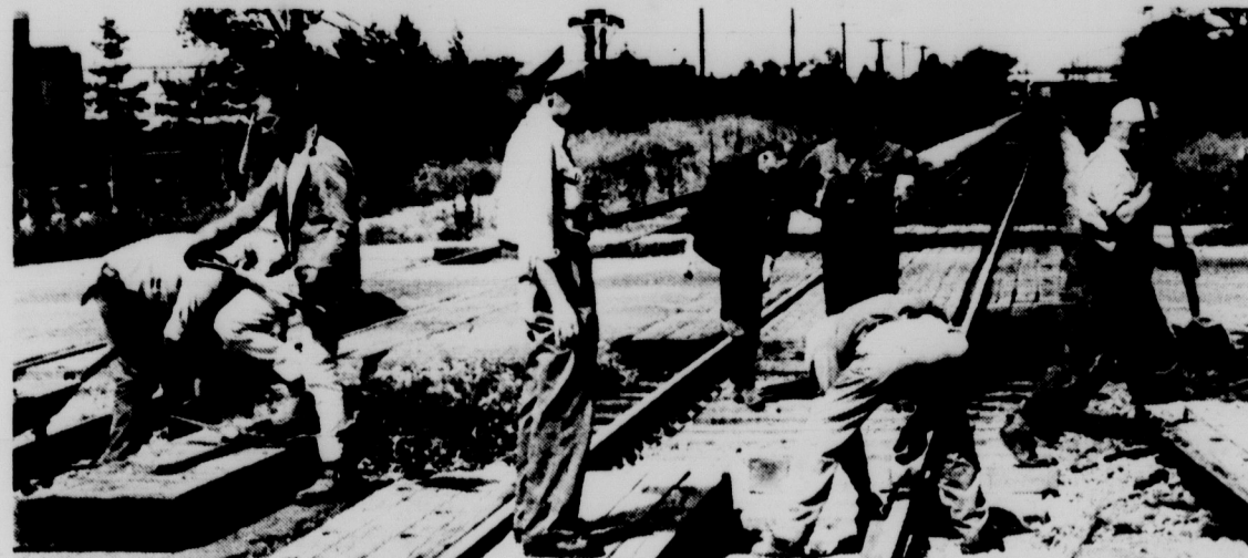
SHADES OF CASEY JONES -- In folk lore, men like John Henry, Joe Magarac and Casey Jones could drive steel, build rails and drive trains with little effort, but it takes a little longer today, as these men can testify. They are working on the crossing on Harrison Road, near Spartan Village. Photo by Patti Prout
