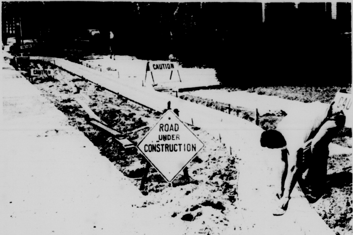
KEEP YOUR EYE ON THE ROAD -- It looks as though some of the workmen concentrated more on the girl in the background than on their work when they built this curb in front of the Home Management Building, but actually it's supposed to curve in. The spot will be a bus stop in the fall. Photo by Ken Roberts
