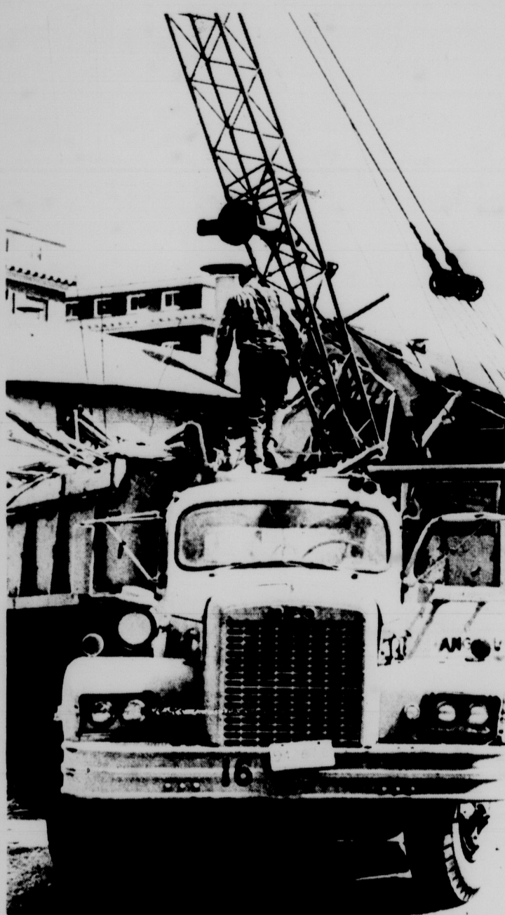
IT AIN'T WHAT IT USED TO BE — The old metallurgy laboratory near Olds Hall is being torn down because of outmoded and insufficient facilities. Here parts of it are being hauled away. Photo by Larry Fritzman
