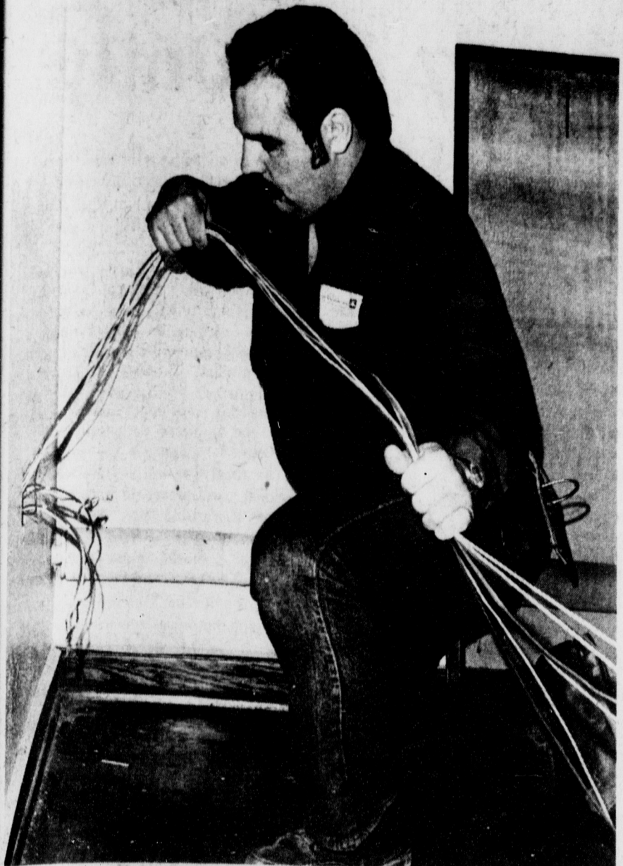
Electrician Gerald Loughlin installs new wiring and electrical outlets in Mayo Hall. Mayo and Landon halls are being repainted, repaired and rewired over the summer break.
